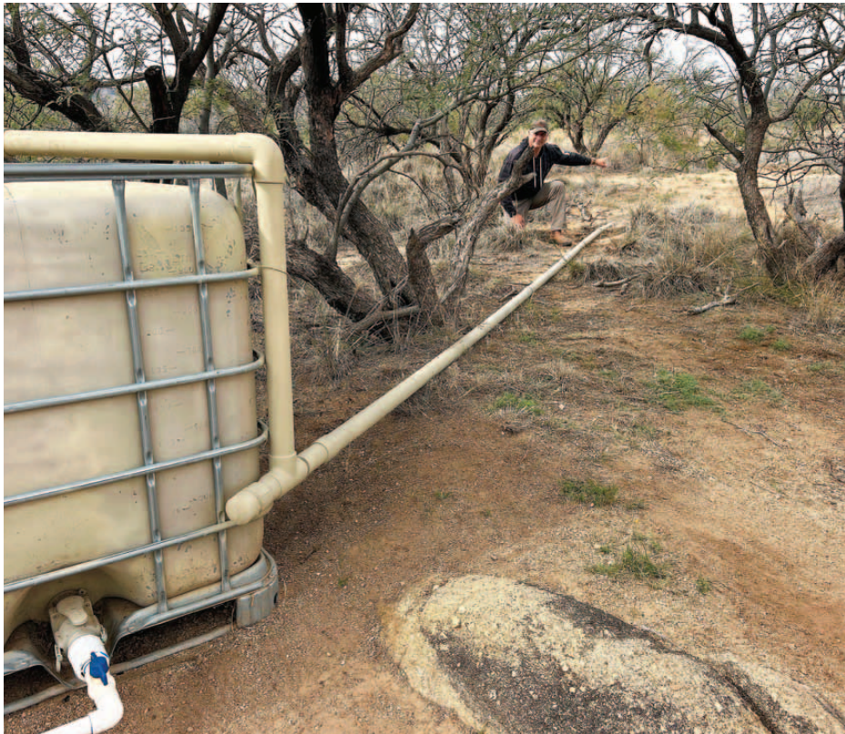
2-inch transfer piping runs 150 feet downslope and empties into IBC storage tanks.
