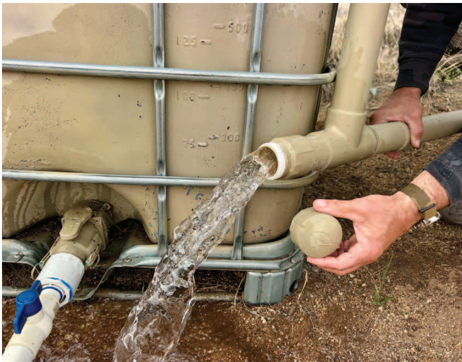
Transfer piping can be drained for freezing weather and cleaning of debris.
