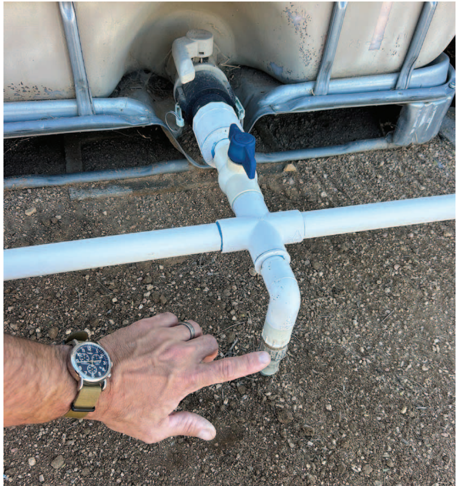
1-inch PVC pipe that connects IBC tanks is connected to 1/2-inch irrigation tubing that proceeds underground to the watering trough.
