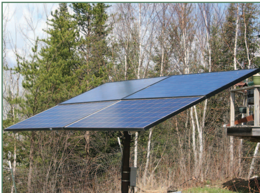
This is our first set of larger solar panels, which gave us more access to power.
