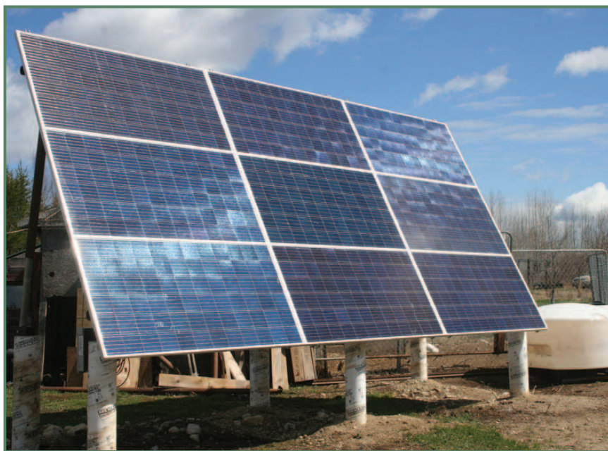
Slowly, we added more solar panels. This is our second array. Will is working on a third in his spare time for the panels we have already bought.
